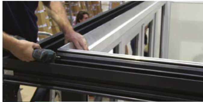
15 Screw the aluminium gutters and the ringbeams together at approx 400mm centres.
