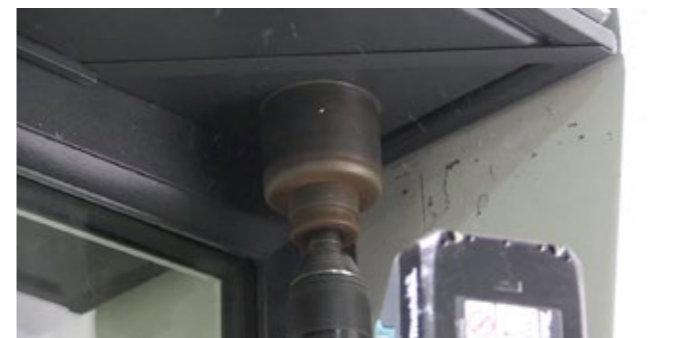
11 Drill a circular hole in the aluminium gutter to create the downpipe outlet.
