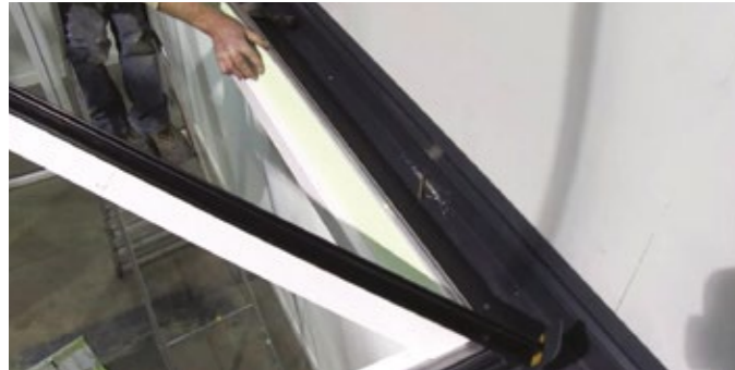
7 Before fixing down the rafters, temporarily fit foam boards against flap to correctly space rafter positions.
