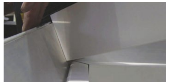
6 Rotate the ringbeam flaps keeping them tight against the hip rafter cut before fixing.
