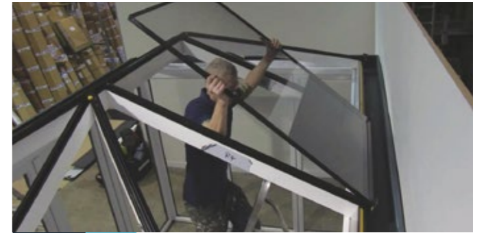
4 Lift glass into place behind the rafter end stops and press down glazing. Make sure the protective yellow tape is removed.
