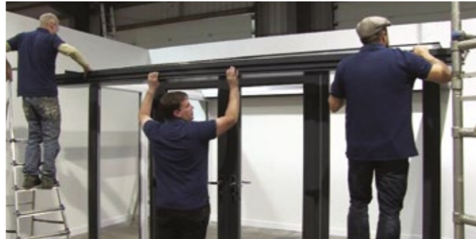
13 Fit the front gutter by hooking it onto the pre-fixed hanger plate.
