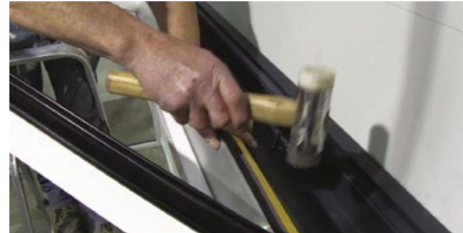
1 Once rafters are fixed, remove the foam boards and locate the glazing shelf.
