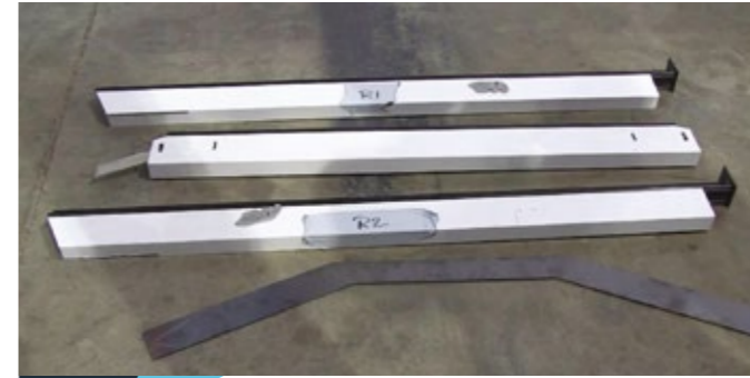
1 Layout the routed ridge, central rafters and tie bars on the ground.
