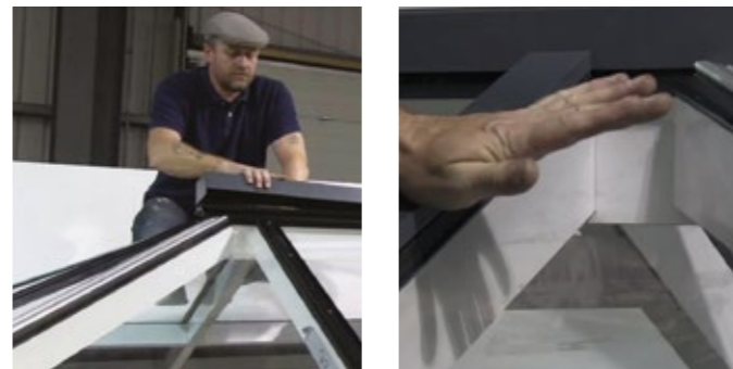
5 Position the ridge cover cap over the ridge pressure plate and clip down securely. Clip on the external cover caps.
